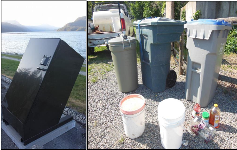
Figure 3. (Left) City Parks staff installed bear resistant garbage bins at Mowat Bay, and at the Complex Bike Park in June as a proactive move to secure garbage and promote public safety. (Right) Garbage cans tested at the Kamloops Wildlife Park during WSBC training in May took less than 10 seconds for bears to break into.
